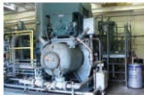
Monmouth Energy's solar turbine recently surpassed 90,000 hours of operation since its last oil change with Mobil SHC 824.
